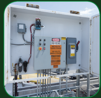
Main Electrical Controls
