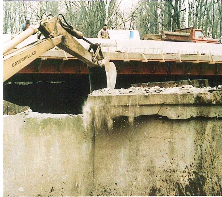
A backhoe quickly topples two ton section off pier top in a few seconds. A new top will be placed on the remaining section to widen the highway from 4 to 6 lanes. Hydraulic splitting method speeds up demolition and reduces costs.
