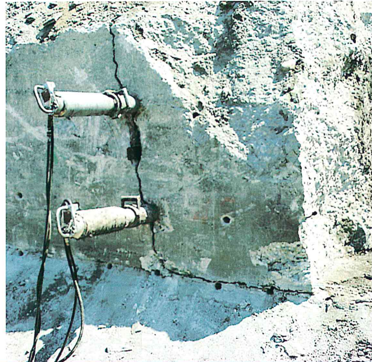
Using two hydraulic splitters, this 8 ft. to 12 ft. thick concrete wall was broken into pieces and removed by a 988 Cat. The contractor speeded up demolition work on this 800 ft. wall many times over other breaking methods.
