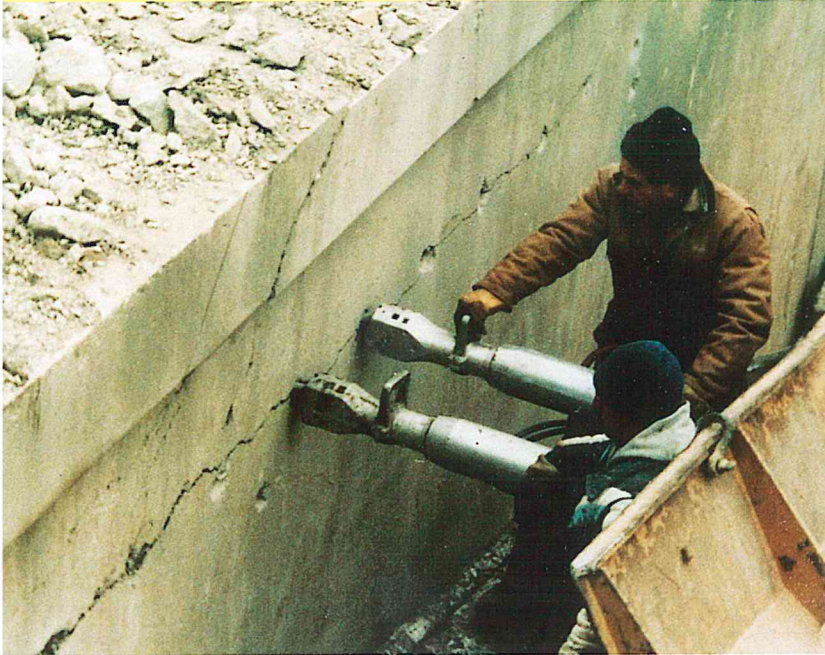
Work crew uses two hydraulic splitters with breaking force of 770 tons to cut two feet off of top of bridge piers. Split was made in less than two minutes along the drill hold line. No impact cracks were left in the remaining lower section to be saved.
