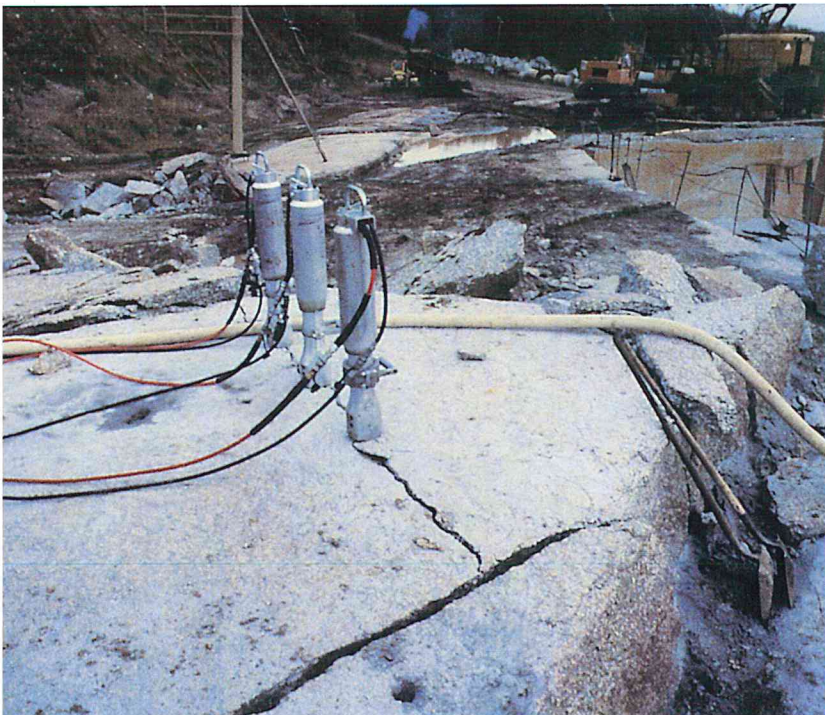
*Three hydraulic splitters powered by a single pump generate over 2 million lbs. (1155 tons) of breaking force to split a 8 ft. x 22 ft. block of granite cap rock in a Midwest quarry. The Elco pump, with manifold, can power 4 splitters if more force is required.
